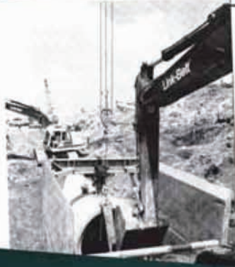
Reeves Ditching and Contracting handled the underground construction of the Georgia Dome project.
